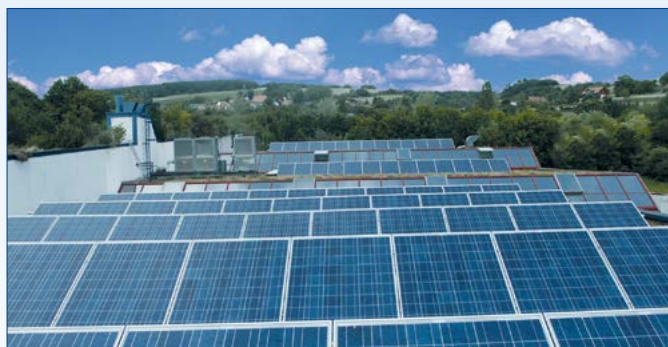
Hevert-Photovoltaikanlage in Nussbaum
